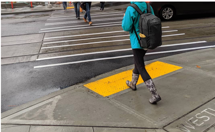
New or upgraded curb ramps at various intersections along N 40th St.
